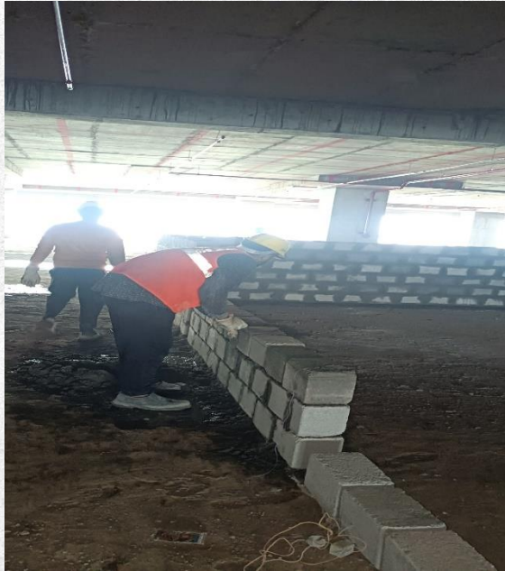
Tower -A L-22nd floor Brick work for electrical and Elv rooms work in Progress
