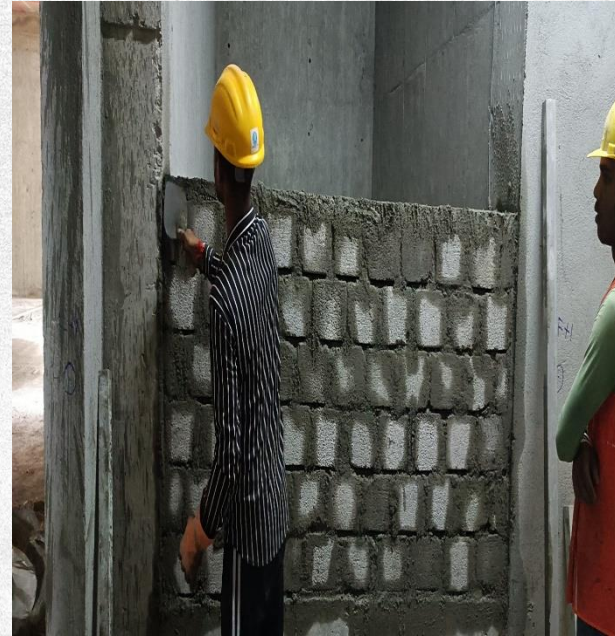
Tower -A L-22nd floor Brick work for electrical and Elv rooms work in Progress
